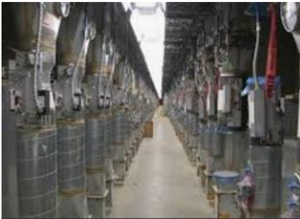
Figure 11 State-of-the-Art White Oak Infrastructure: Advanced Air Terminal Units Supporting Laboratories
